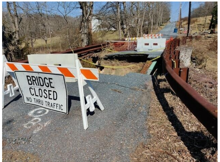
Bridge out on a road paralleling Rt 202. Not much chance is jumping this one!
